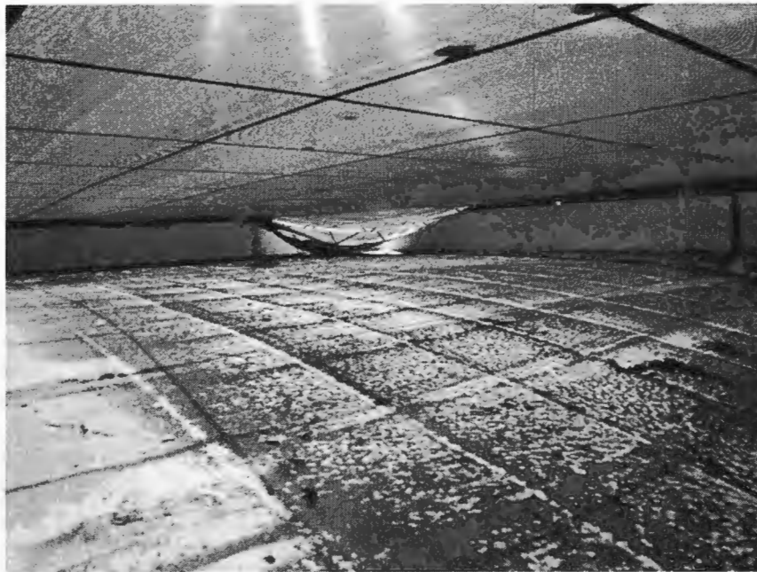
Figure 3 – Subject Pool Shell (Empty due to suspected leak in deep drain line)
