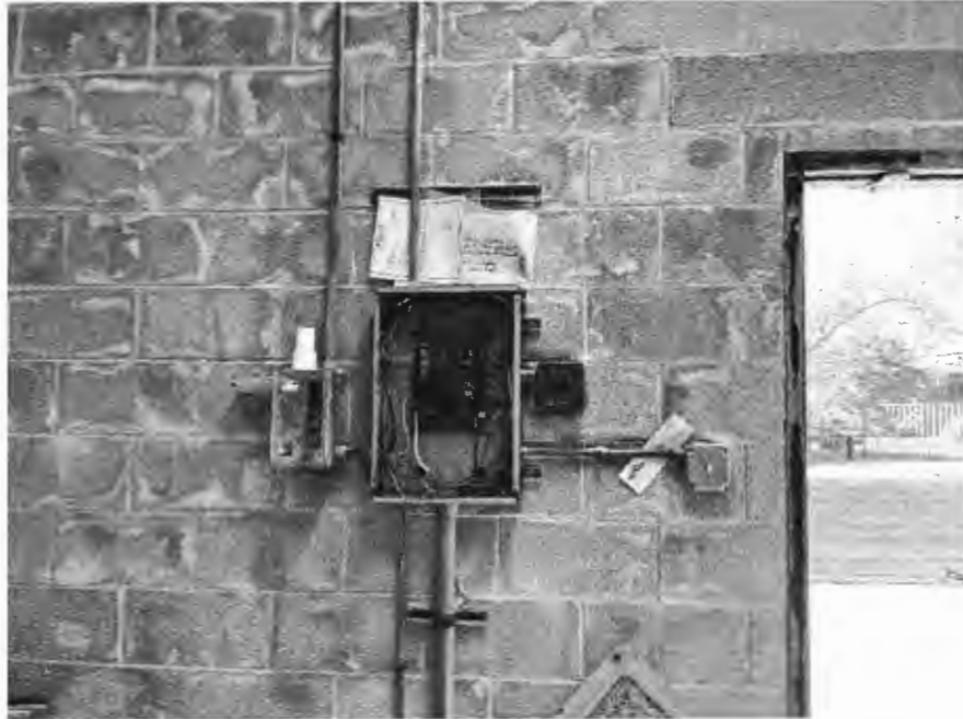
Figure 4 – Electrical Panel with Corrosion and in a State of Disrepair – Note efflorescence or chemical staining on walls
