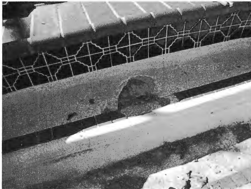
Figure 1 – Area of plaster in a state of disrepair
